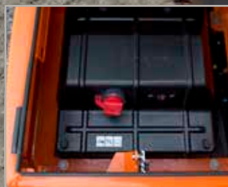
Battery cut-off switch
